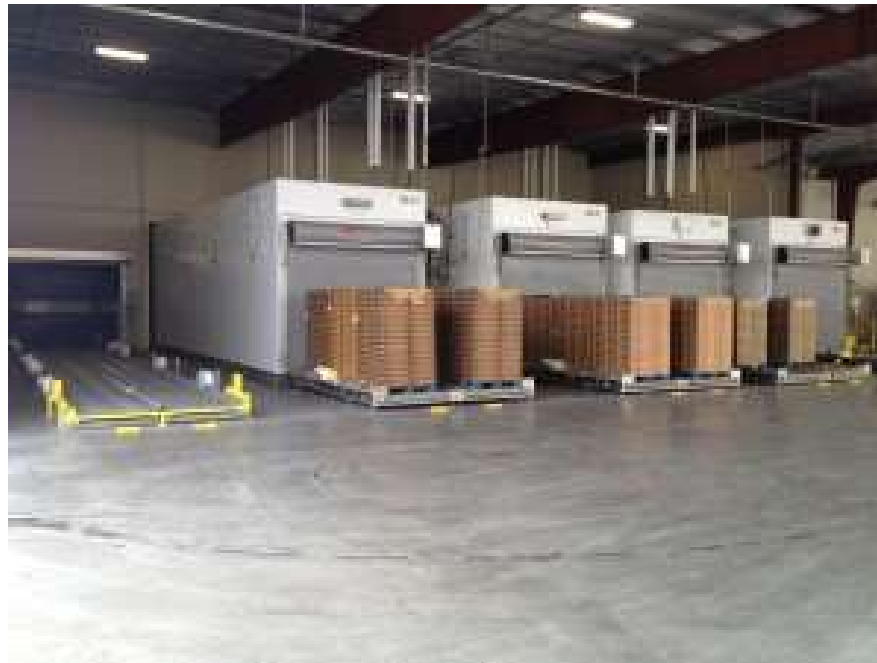
MACS Coolers, Castroville, CA
